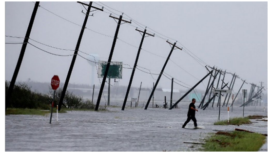
Damage to electric infrastructure in Texas. Source: Adrees Latif/Reuters. 218
