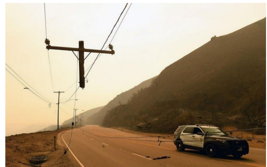
Damages to electric lines along the highway. Image Source: Alejandra Reyes-Velarde | Los Angeles Times. 140
