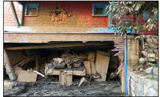
Gas crews work a damaged line after an RV was carried by the mudslides into a home. Source: Roa. 174
