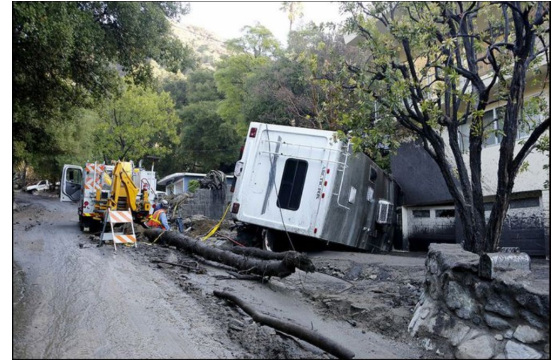
Damage to a home on Country Club Drive in Burbank, CA. Image source: Rob Kay/ICF.
