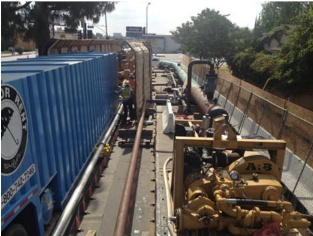
Figure 12: Hydrotest Set Up with Sound Proofing to Minimize Noise Complaints (located behind Baker tank)
