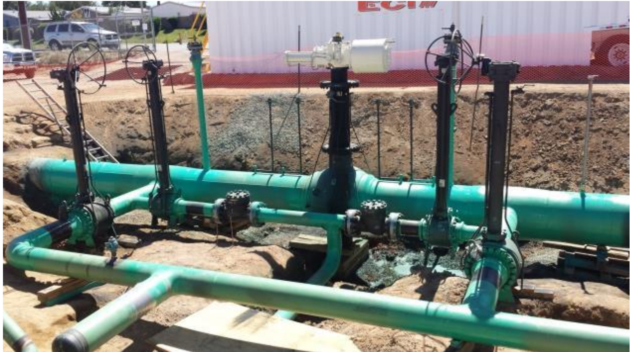
Figure 7: Assembly for L235W at Palmdale Tap: 30" MLV 235-215.22-0 shown with new actuator (in white) along with [redacted] bridle valves to and check valves to SL 44-654; [redacted] blowdown valves are also shown.
