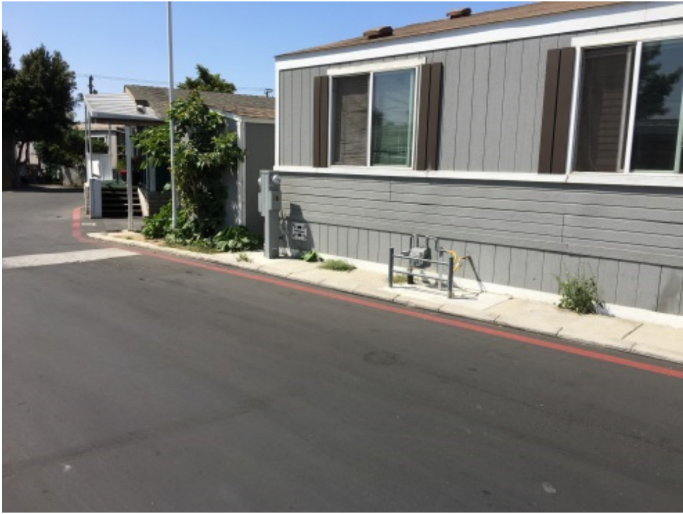
Fig.7: Newly installed utility meters at the front of a mobile home lot installed in accordance with current safety standards
