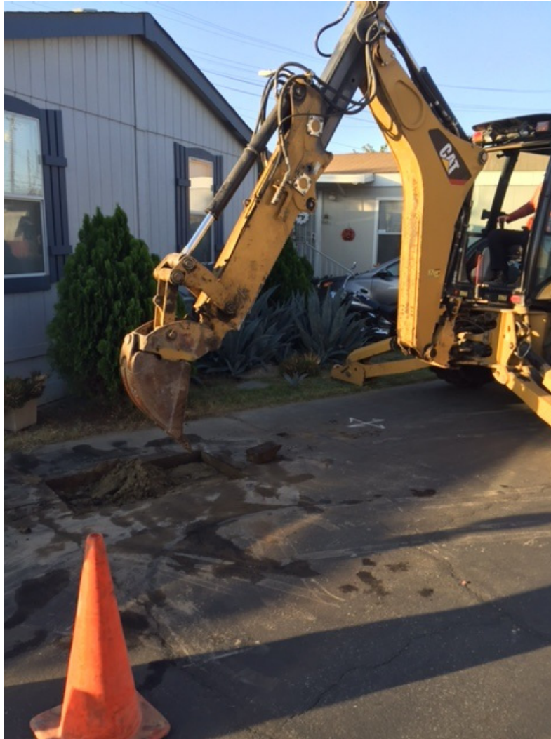
Fig. 1: Contractors must pothole the MHP prior to full commencement of construction. This minimizes the risk of striking existing utility lines.
