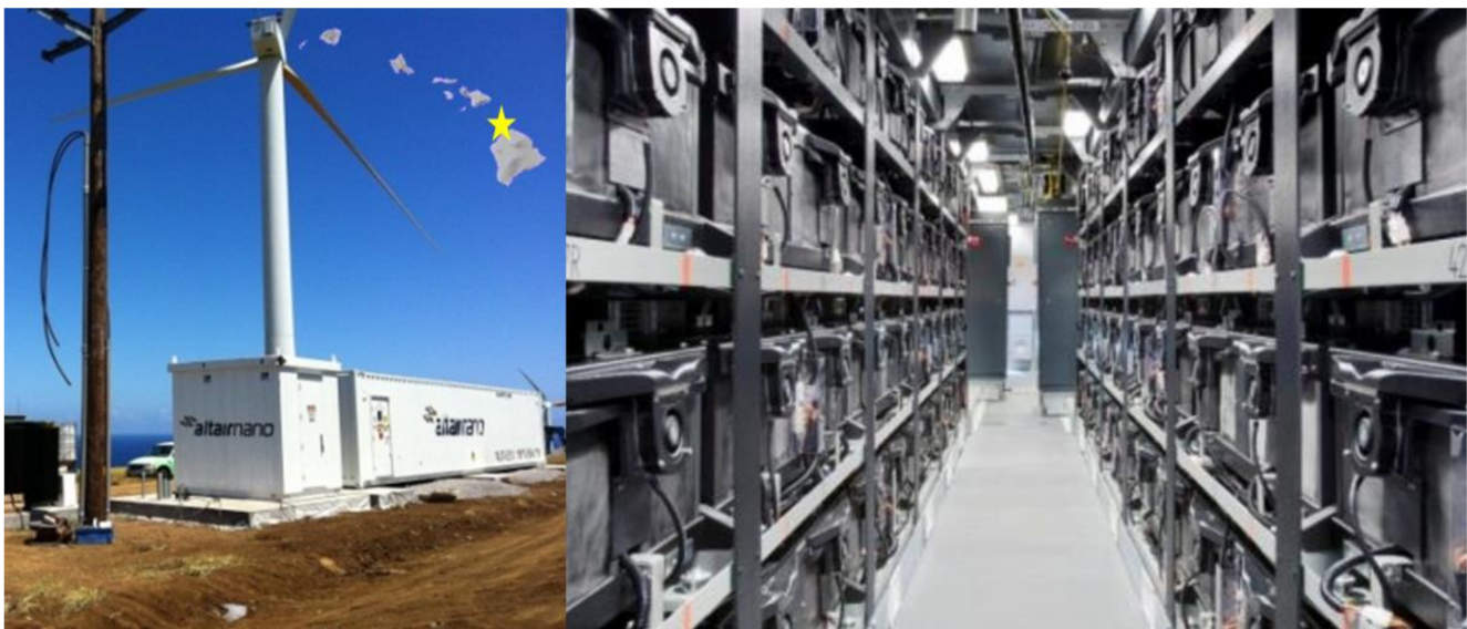
Figure 1. Outside and inside view of the BESS.
