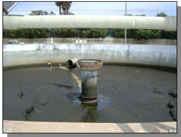
One gravity thickener is used to thicken the primary sludge.
