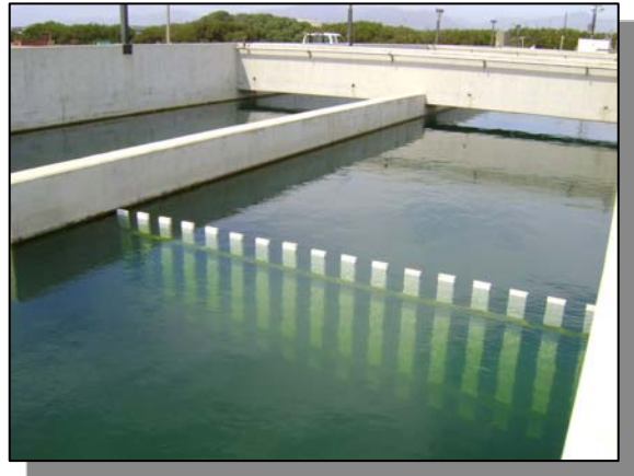
Baffles located in the chlorine contact tanks prevent short-circuiting.
