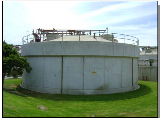
The Ventura WRF has three anaerobic digesters.
