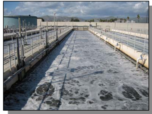
The Ventura WRF has four aeration basins operated in series.
