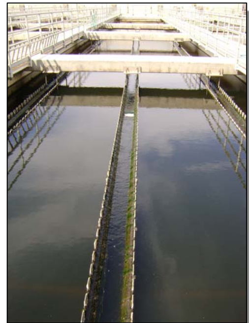
One of the six rectangular secondary clarifiers.
