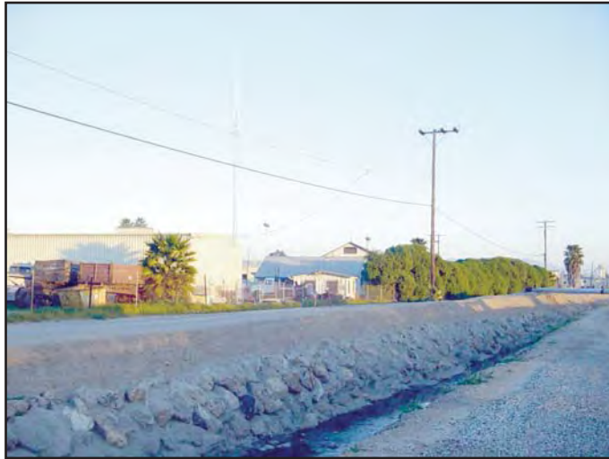
Photo 1 View of concreted rip-rap that lines the banks of Brown Barranca in the Saticoy District.
