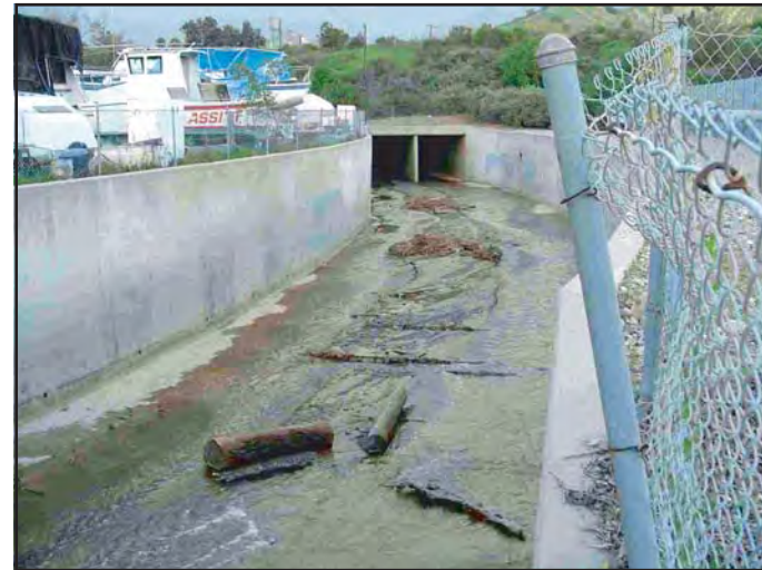
Photo 4 East of Ventura Avenue, Cañada Larga Creek has been channelized with concrete banks.
