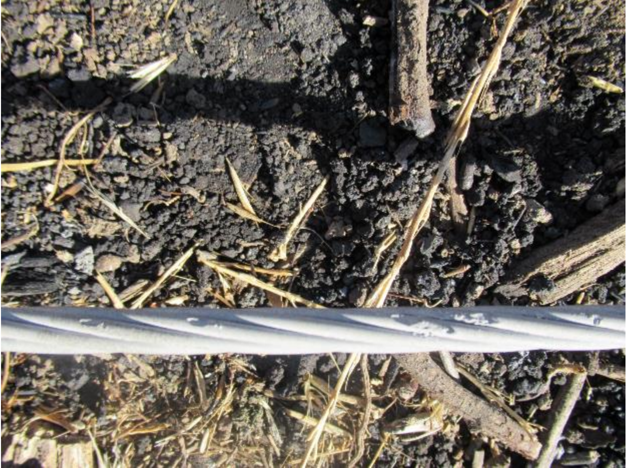
Figure 10: SED photo of Anlauf Canyon site, pitting on the east conductor between poles numbered 3002114E and 1202085E.
