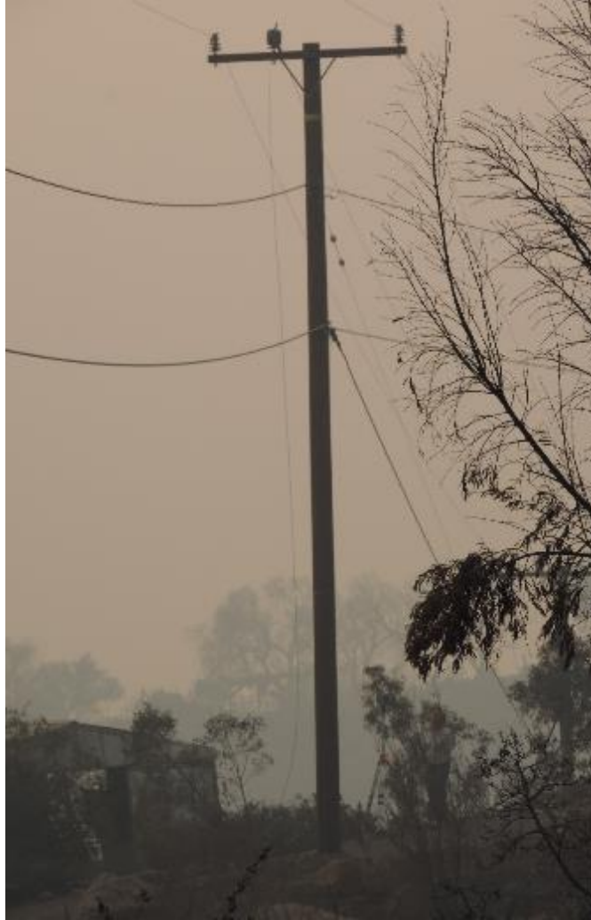
Figure 3: SED photo of Koenigstein site, 729565E with center primary conductor laying on the ground.
