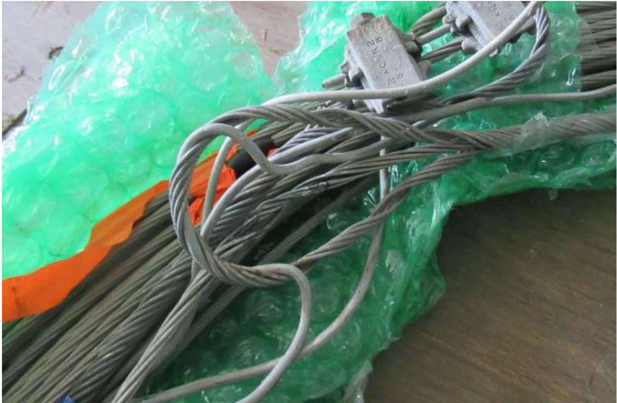
Figure 14: SED photo of February 2017 Anlauf Canyon evidence examination, arc marks and bird-caging on the east conductor between poles numbered 1025341E and 3002114E.
