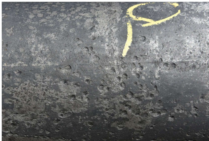
Figure 90: Type II Corrosion—Isolated Small Pits
