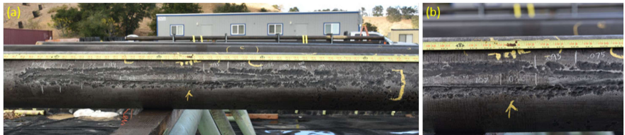
Figure 32: Pipe Body Corrosion on C020
