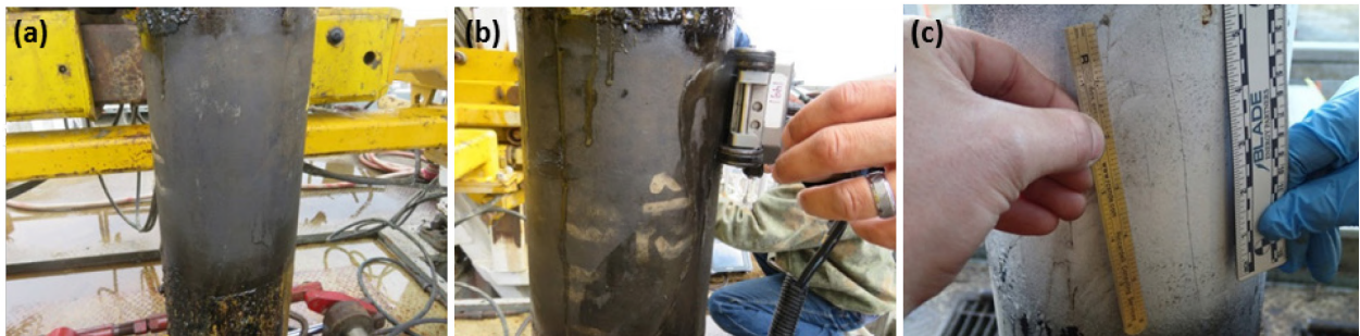
Figure 45: (a) Cleaned Pipe Section for NDE, (b) Ultrasonic Transducer, and (c) MPI Linear Indication
