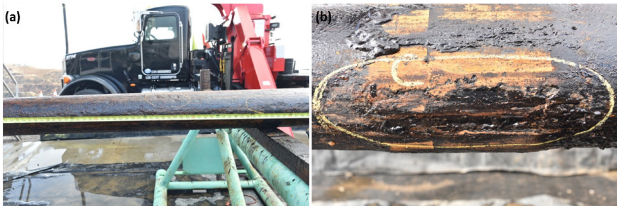
Figure 48: Corrosion Features on C018 (a) Pipe Body and (b) Connection
