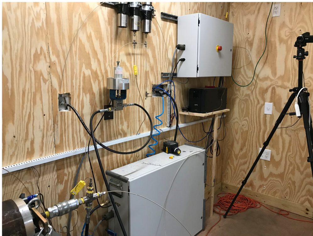
Figure 11: Inside the Conex—Pressure Cabinet and Control Box
