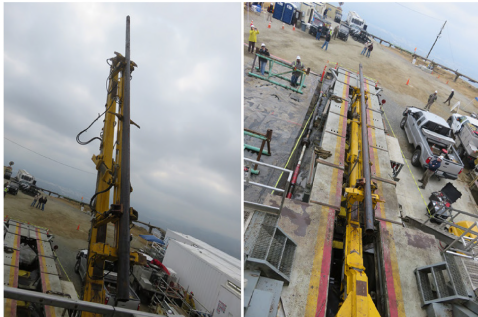
Figure 47: Casing Pipe Handler
