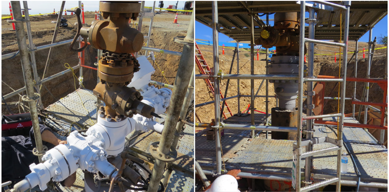
Figure 20: Wellhead Magnetic Particle Inspection
