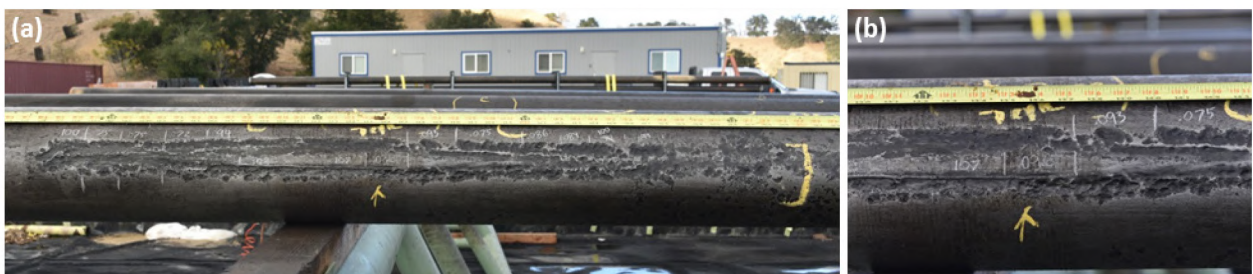
Figure 57: Pipe Body Corrosion on C020
