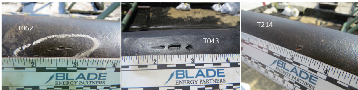
Figure 33: Examples of Mechanical Damage
