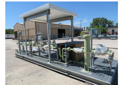
Gas Blending Skid
