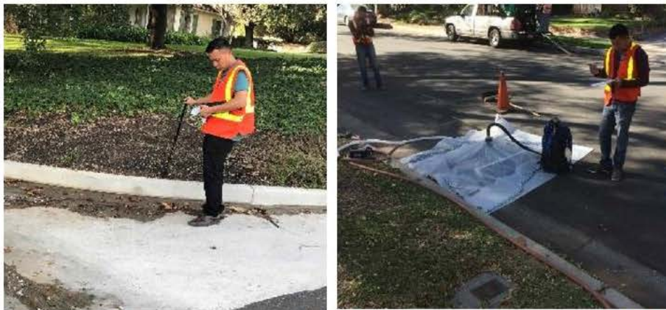
Figure 1. Leak Site Prescreening (Left), Surface Expression Measurement (Right)
