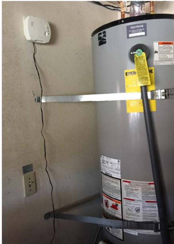
Residential Methane Detector installed adjacent to gas water heater
