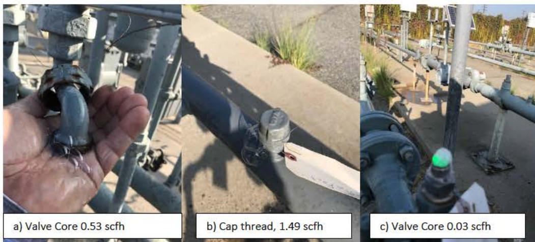
Figure 4. Simulated/Controlled Leaks (a) and (b), (c) Actual leak detected and located by sUAS leak survey and verified by ground crew.
