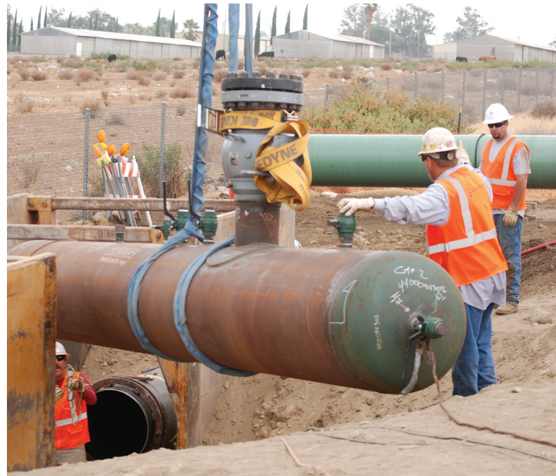
Work crew members guide a test head cap into position at one end of a pipeline segment to be pressure-tested.
