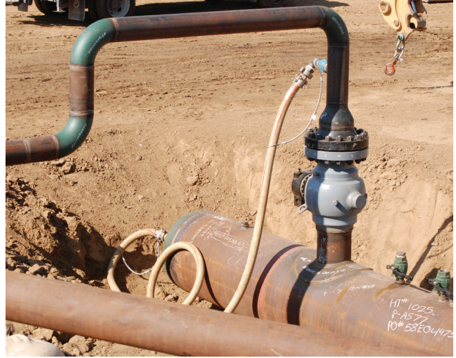
Water is pumped into a test head to conduct a pressure test.
