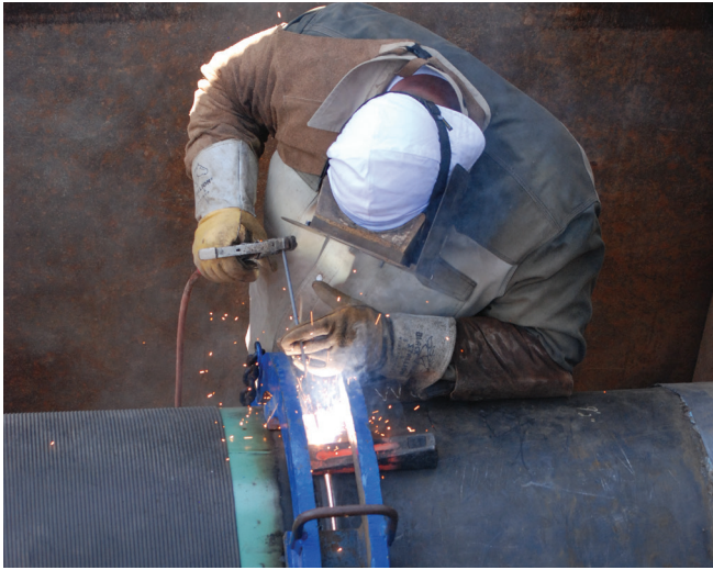
A pipeline test head cap is carefully welded to the end of a pipeline segment to be pressure-tested.
