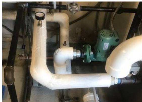
C.E. Mechanical is a full-spectrum mechanical services contractor that works with SoCalGas to obtain boiler, pipe insulation, and other rebates for the benefit of its customers.
