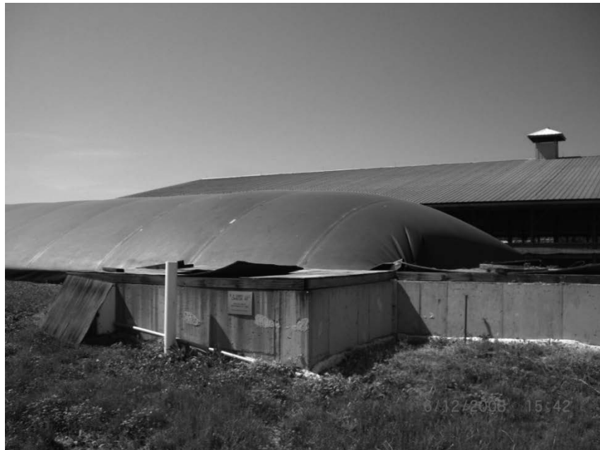
Photo 3-1—AA Dairy Digester in Operation
