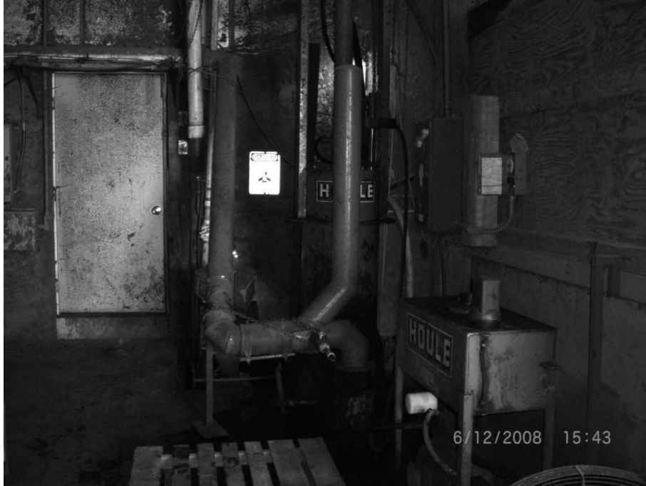
Photo 3-2—Houle Piston Pump Used to Deliver Raw Manure into the Digester
