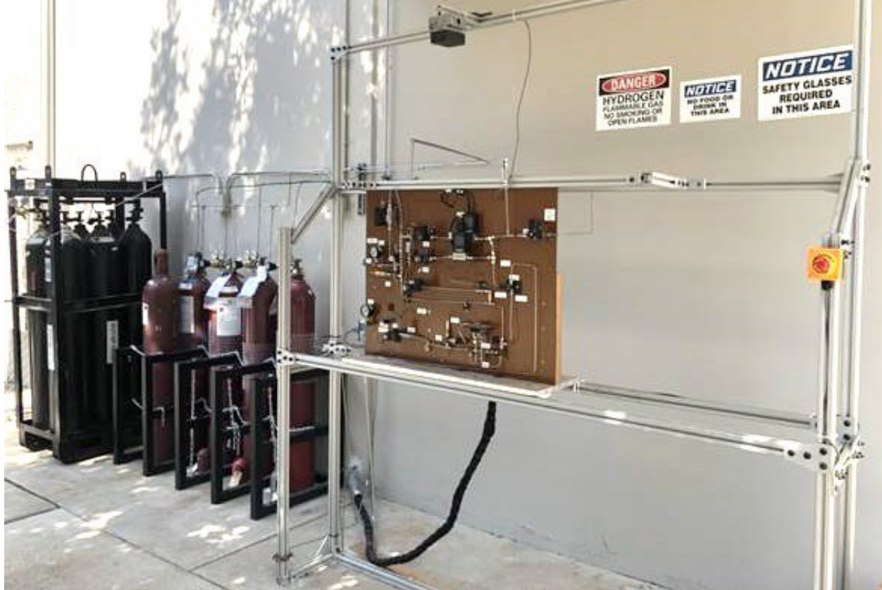
Figure 16: Controlled Gas Leak Testing Instrumentation Setup
