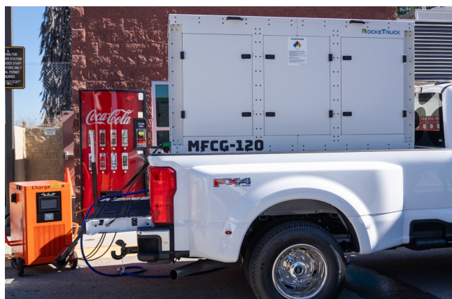
Figure 5: Pickup-mounted RockeTruck “Mini” Fuel Cell Generator at CSULA Demonstration
