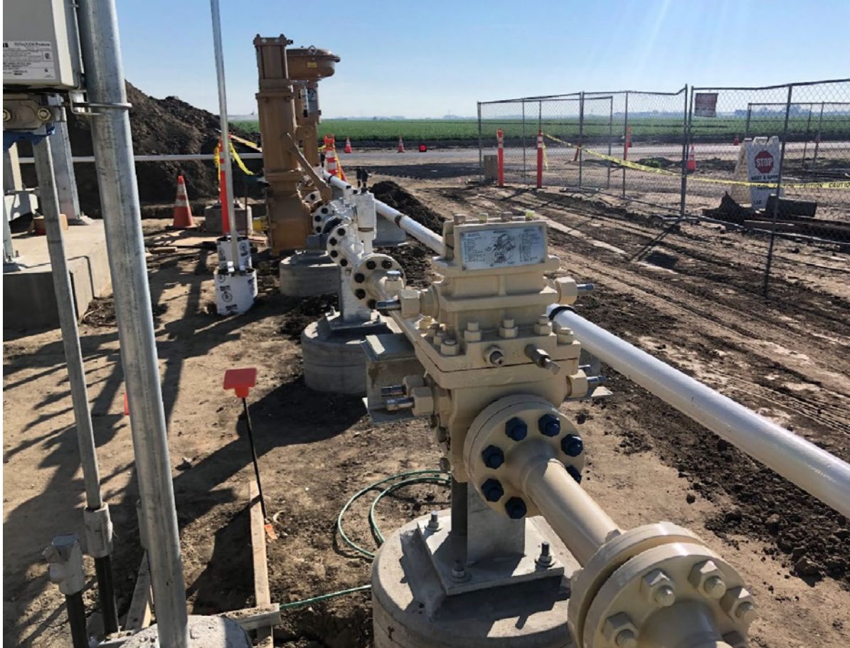
Figure 7: Facility Equipment and Piping
