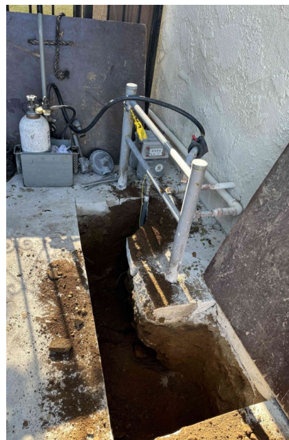
Figure 6. Houseline placed on Natural Gas Tank
