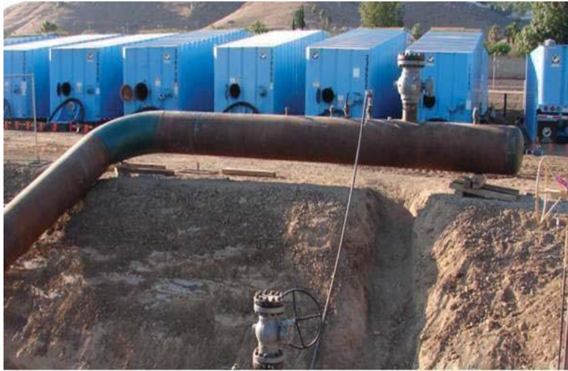
Figure 26: Water Tanks and Test Head
